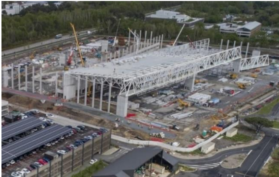
Mérignac / multipurpose production building
